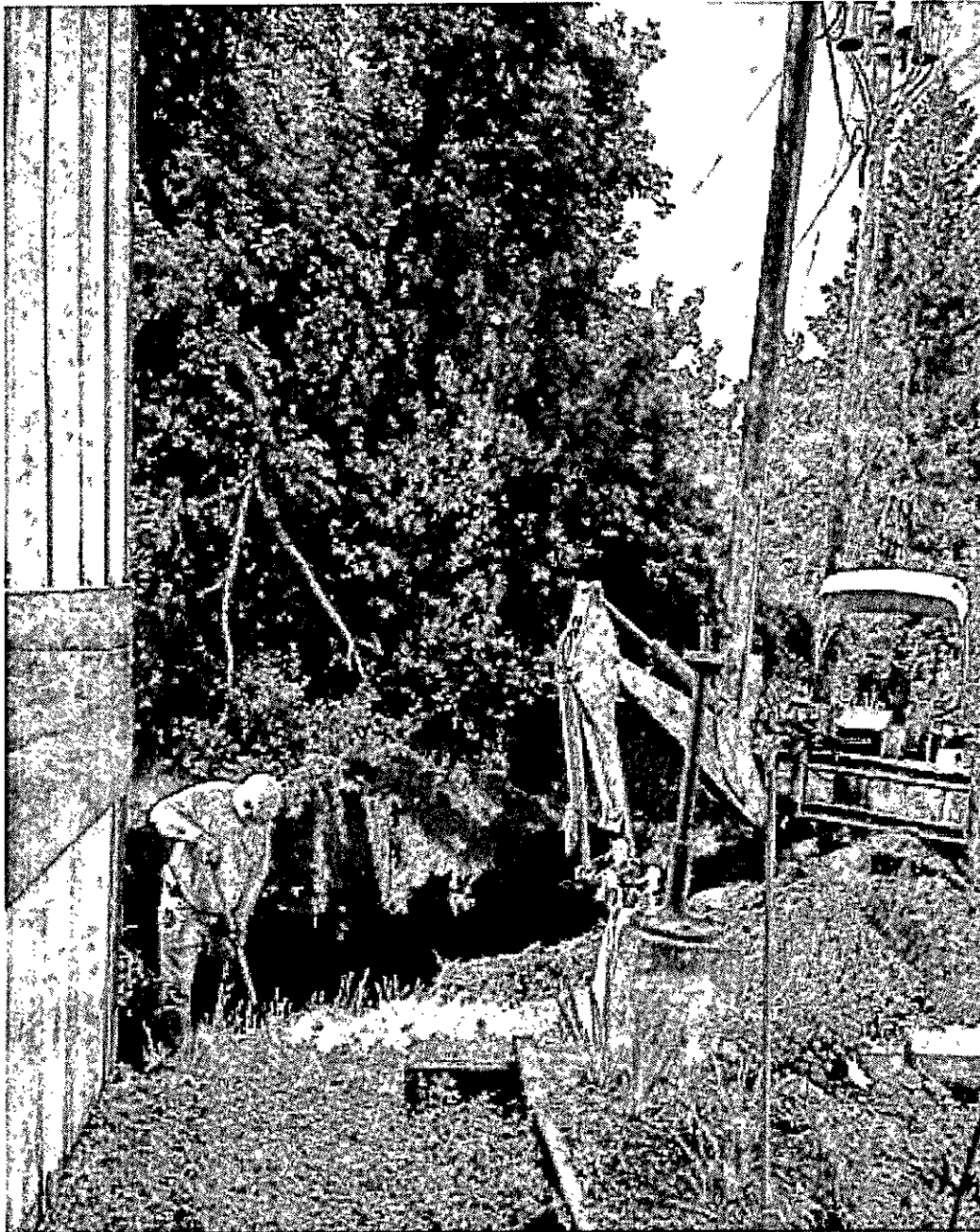
Figure 26. Historic Depot laying electrical power lines from utility pole to service panel inside of the Finlayson depot.
